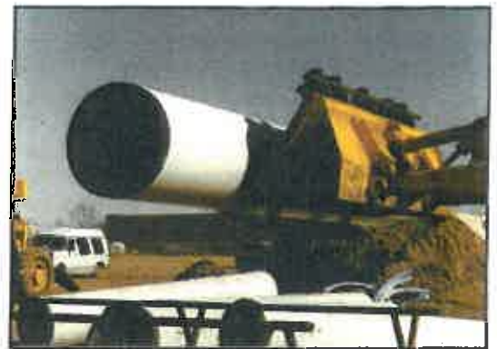
Lightweight, 15-ft. long Vylon Slipline joints are easily handled and staged for insertion.
