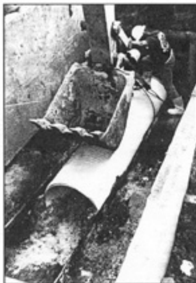
Backhoe bucket maintains control of new joint prior to assembly. Contractor poured concrete mats for work area floor safety and to keep dirt out of the line.
