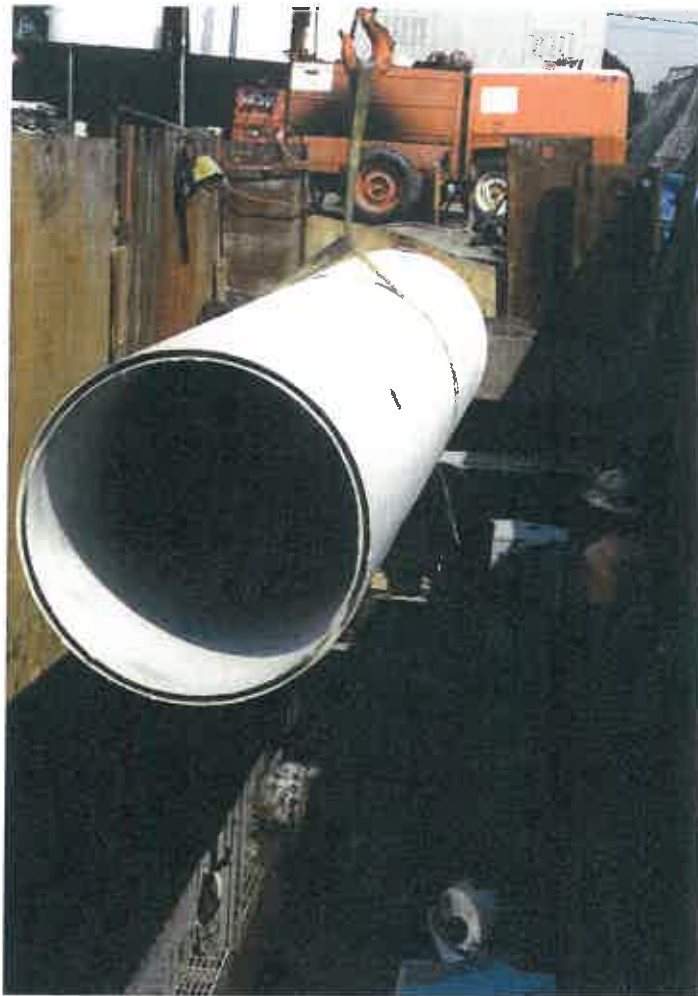
The District 5 Trunk Rehab Project uses 15-ft segments of the 36-in. closed profile-wall PVC sliplining pipe.
