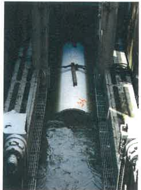
The sewer flows continue uninterrupted at 20 to 80 percent flow capacity during the sliplining process.
